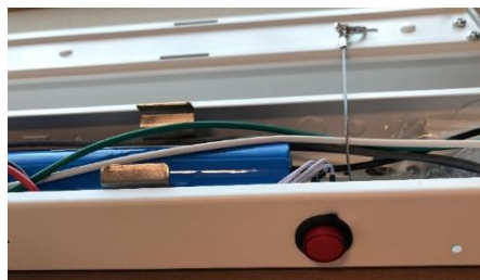
Emergency Test Button
